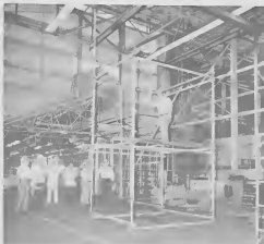
Joe Williams, shown on scaffold platform, demonstrates how easy it is to build a neat structure from prefabricated material. Joe Williams, aki ariba plataforma di stelashi, ta demostra com facil ta pa traha un estructura bon cu material prefabricá.
